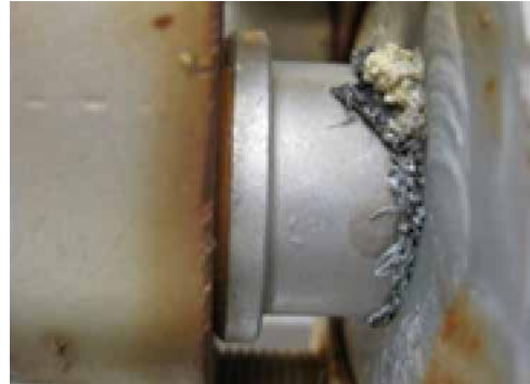
Figure 2: Improper installation: packing out stuffing box
