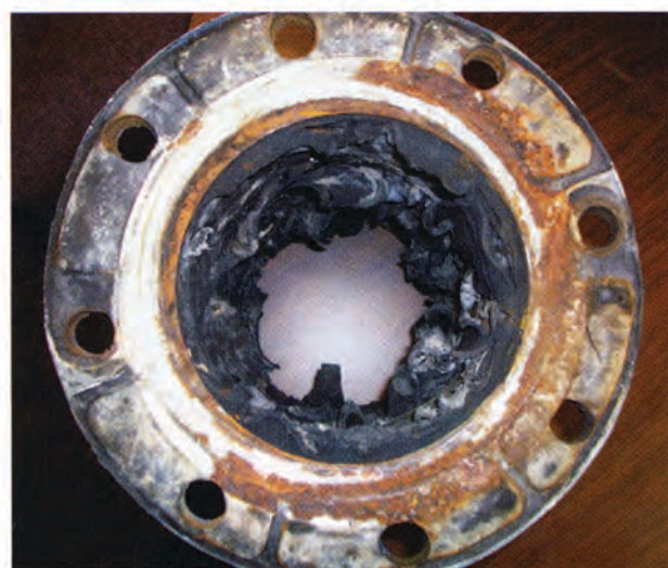
Figure 3: Excessive heat caused the tube in this expansion joint to harden and crack under movement. Courtesy: Garlock Sealing Technologies
