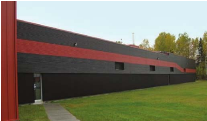
Installation of this solar heating wall slashed natural gas consumption by more than 20,000 cubic yards per year.
